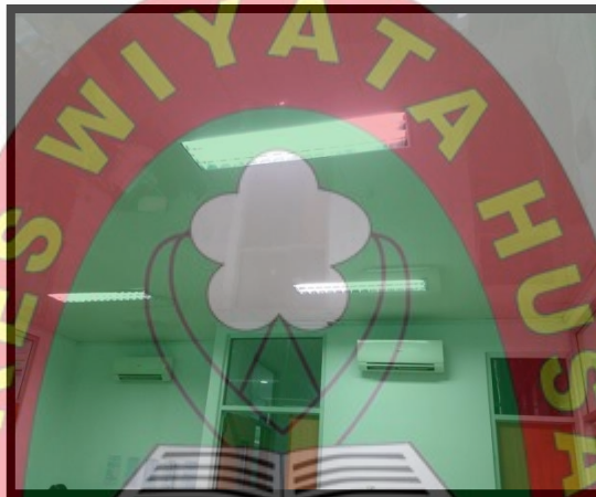
Gambar 2. AC (Air conditioner)
