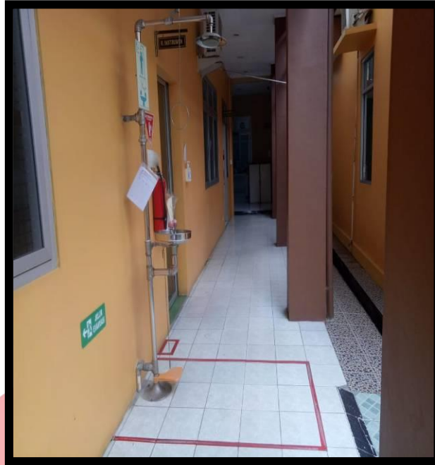
Gambar 11. Pemancar air ( emergency shower )
