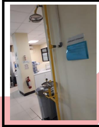
Gambar 13 Emergency Shower dan Eyewash
