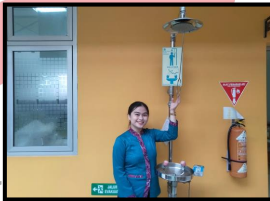
Gambar 3. Pemancar air ( emergency shower )
